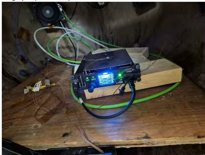
Photo 9 – UUT Operation Verification (3)
